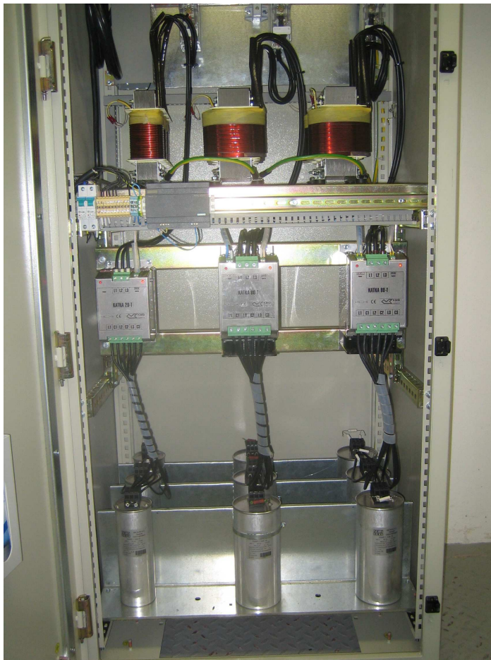
Figure 6: example of three-bank compensation, one KATKA 20T 25 kVAr + two KATKAs 80T, 45 kVAr
